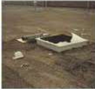
A fatality occurred here!
